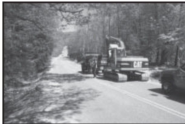
The Public Works Department has been busy with maintenance work projects on Raymond Hill Road and Spiller Hill Road.
