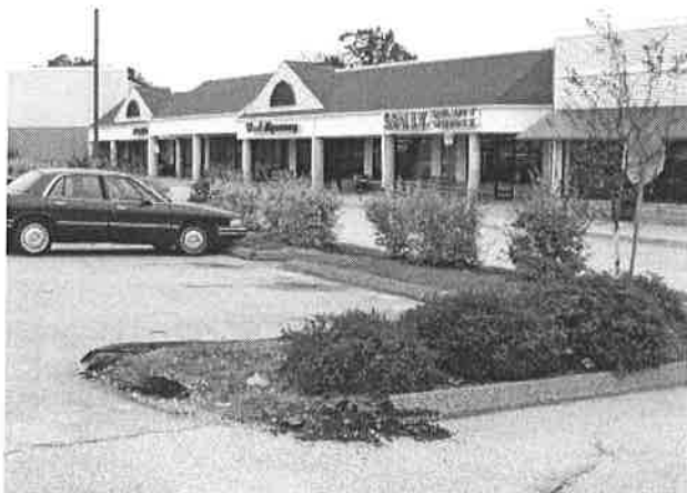
While asphalt curbing is inexpensive to install, it is very prone to snowplow damage.
