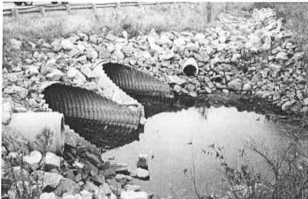
Rip-rap is often necessary to control erosion and stabilize slopes. In highly visible areas, a more refined appearance – accomplished through the use of handplaced stone and/or ground cover – is necessary to avoid situations such as this.
