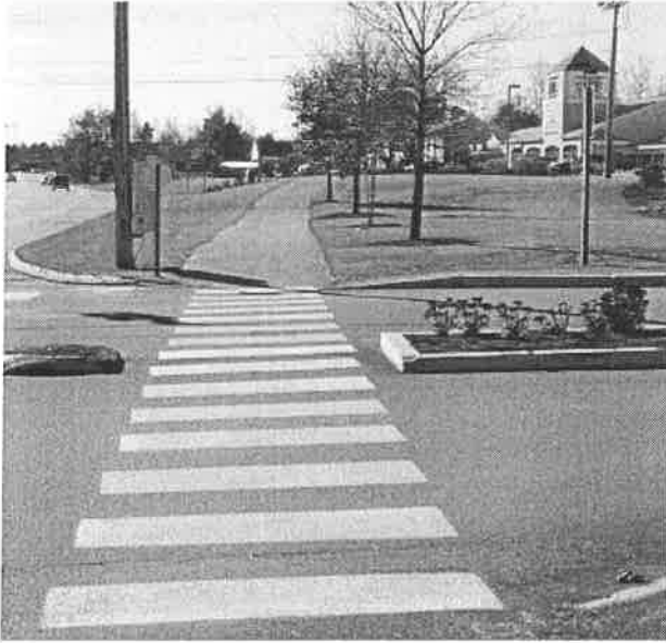
An island provides a refuge zone for pedestrians crossing this wide driveway. Permanent crosswalks should have been used to minimize annual maintenance.
