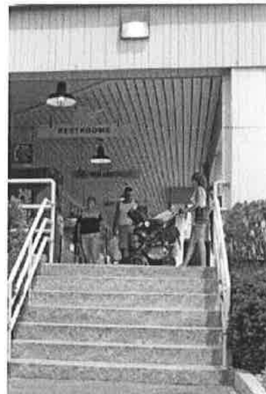
Unshielded wall-pack lighting can cause dangerous glare and make it difficult to see the stairway.
