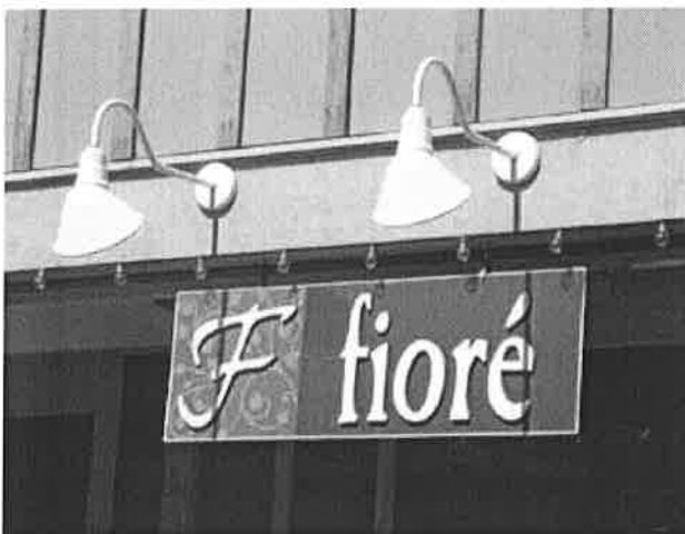
These facade-mounted lighting fixtures are visually compatible with the form and color of the building.
