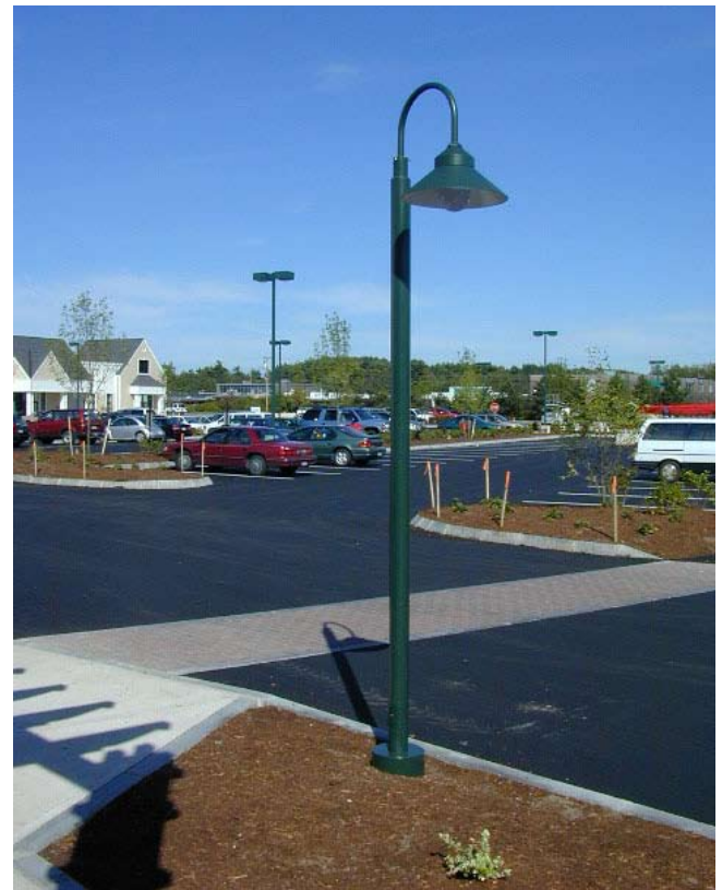
Pedestrian scaled lighting used to illuminate a crosswalk.
