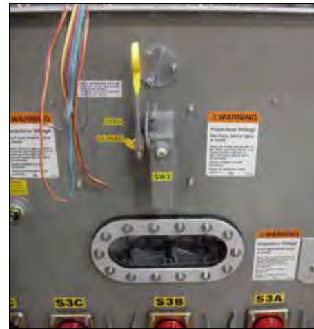
Figure 8. VFI transformer with visible break.
