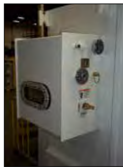
Figure 7. External visible break with gauges.
