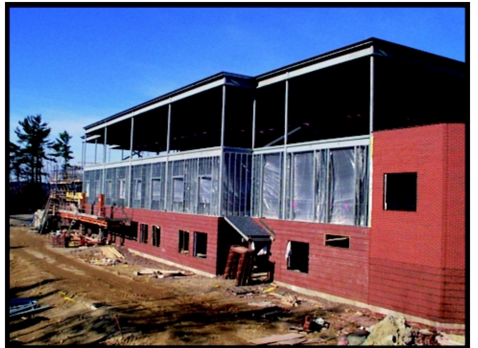
Progress is made on the Raymond Elementary School while the weather is favorable.
